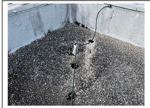
Lightning Protection Downlead
