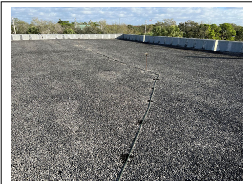
Lightning Protection on Roof
