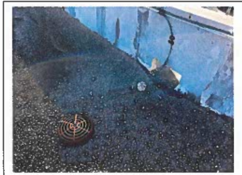
Lightning Protection on Roof & Parapet
